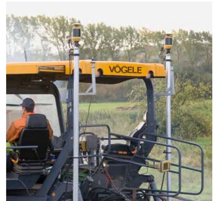
The screed's position and elevation can be controlled and monitored precisely with GPS and laser receiver, for instance.
