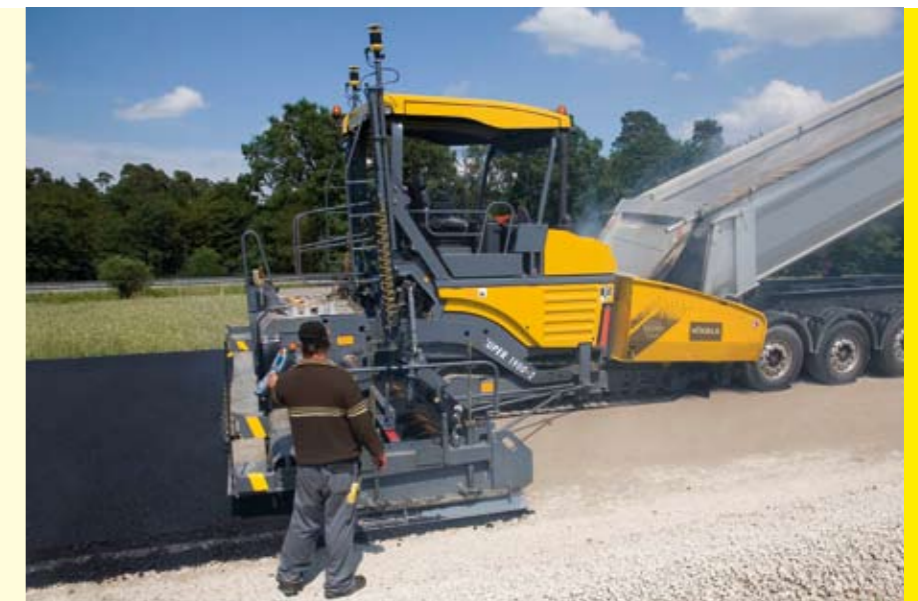
Just like the paver operator, the screed operator, too, can focus his attention on the process of paving and its results. Grade and slope as well as the pave width are controlled fully automatically by the 3D system.
