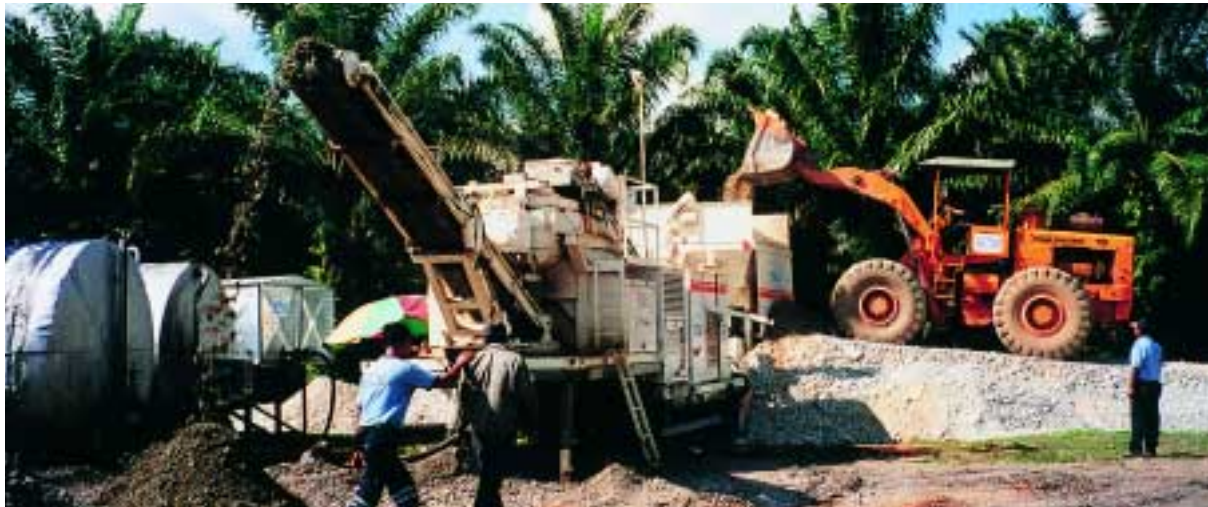
Cold treated material with excellent storing capabilities thanks to a binding agent called foamed bitumen: Here in Malaysia, high-quality base course material was produced with the KMA 150.
