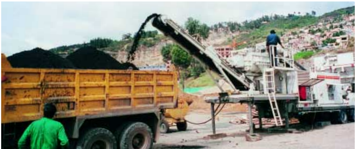
A truck is filled within a very short time: The mobile mixing plant KMA 150 impressively demonstrates its power here in Colombia.
