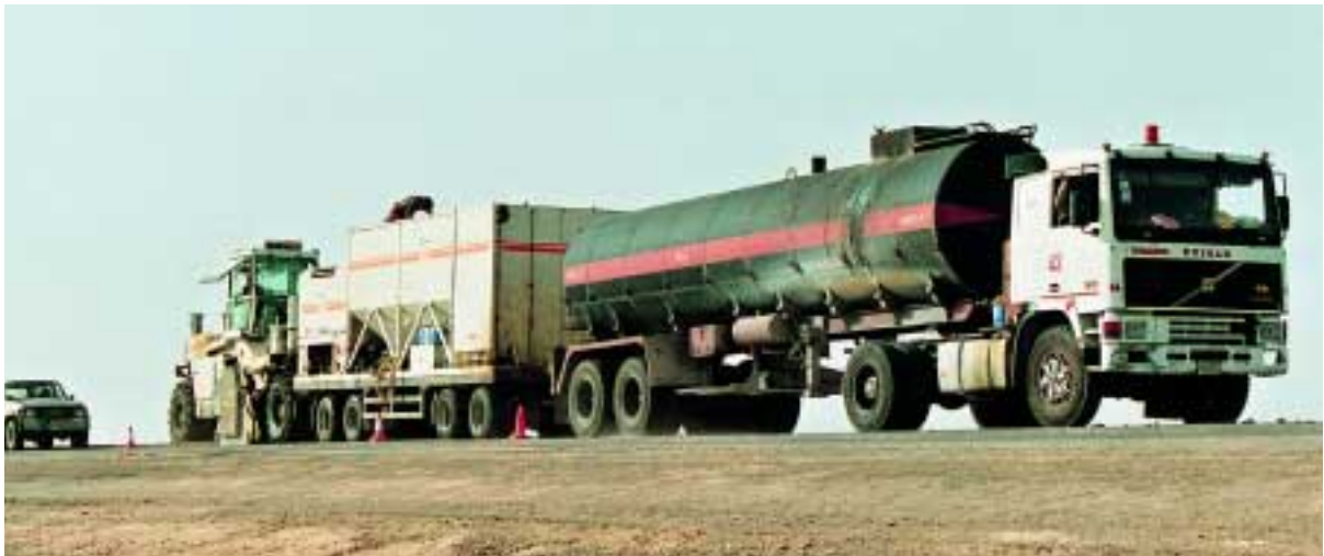
The Wirtgen foamed bitumen technology is a reliable rehabilitation method even in the desert: The recycling train is in continuous operation in Saudi Arabia on a total road length of more than 380 km.
