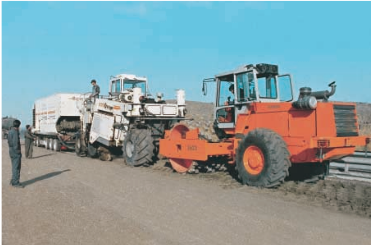
Cold recycling “to perfection”: The Wirtgen WR 2500 demonstrating its power during the rehabilitation of the Teheran-Qom Highway job site.
