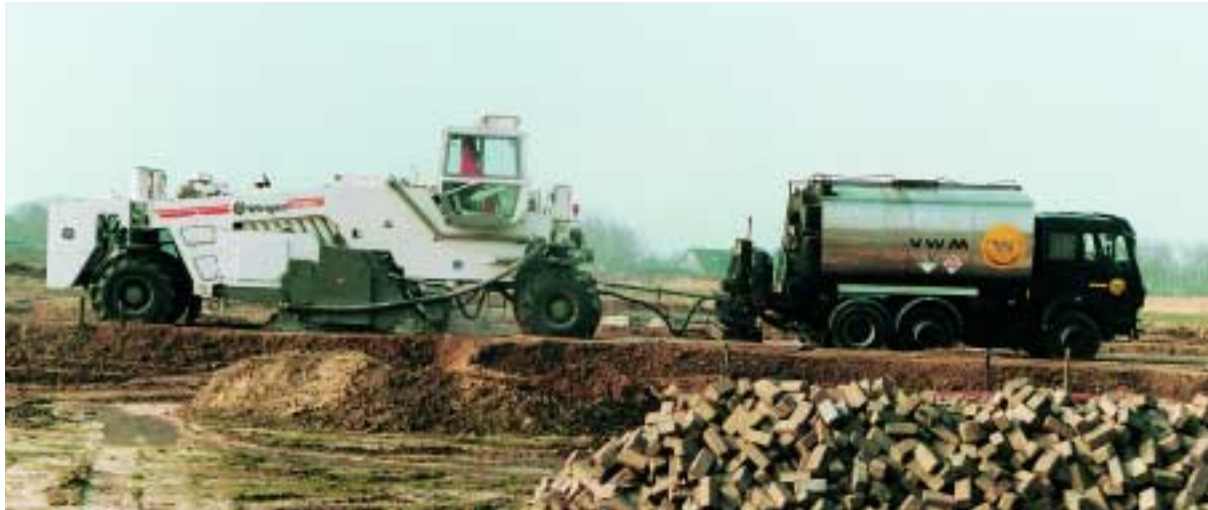
A road rehabilitation project in the Netherlands: The Recycler WR 2500 pushes the insulated bitumen tanker truck in which the hot bitumen is stored.
