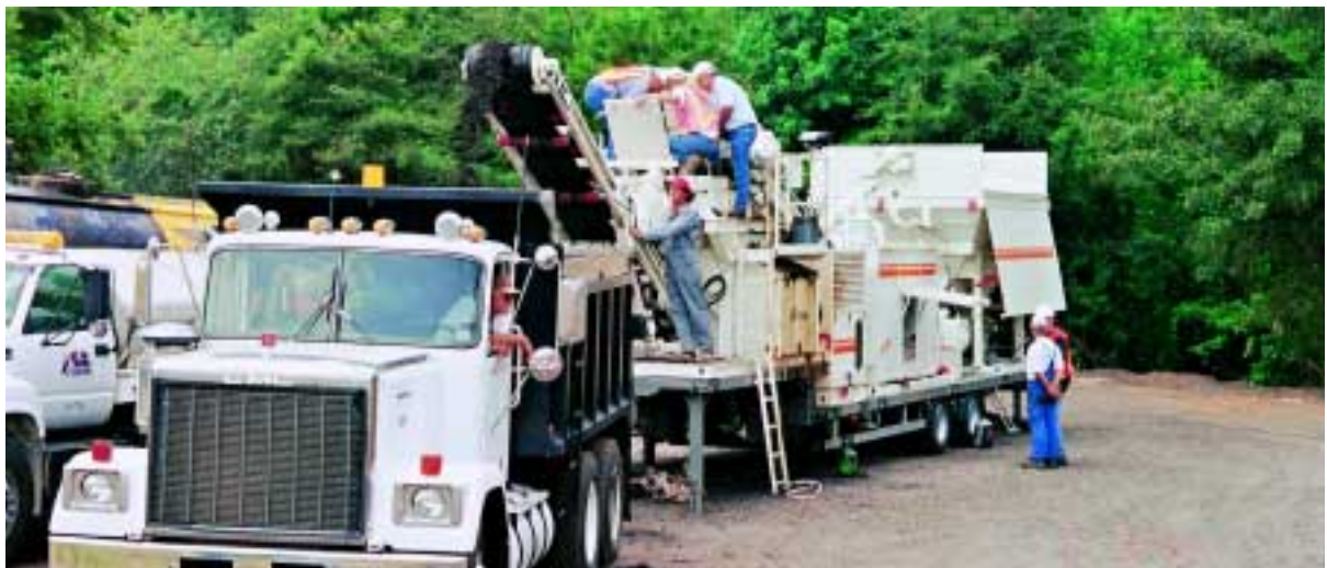
The cold treated material produced by the mobile KMA 150 is loaded onto trucks: In Texas/U.S.A., too, the good quality of material produced with foamed bitumen is well-known.
