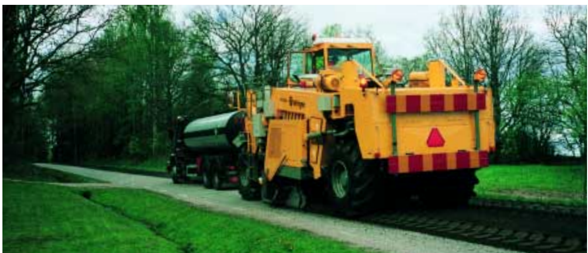
Environmentally friendly road rehabilitation with foamed bitumen in Sweden: The recycling train with the WR 2500 vouches for the swift rehabilitation of damaged traffic routes.
