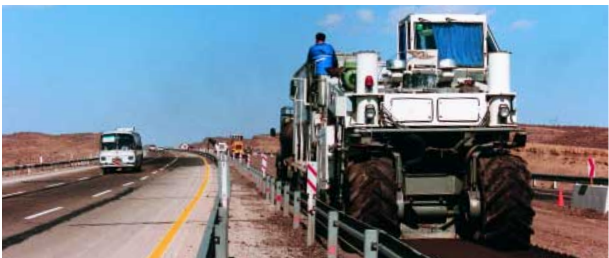
During the rehabilitation of a motorway in Iran, the WR 2500 could once again demonstrate its power: The machine went to work after parts of the base course had been milled off.
