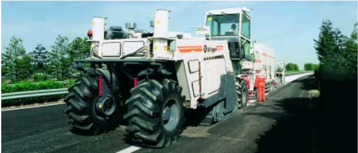
Recycling “in-situ” under traffic is no problem for the WR 250: The “moving job site” minimises traffic obstruction and leaves behind a high-quality base course layer.
