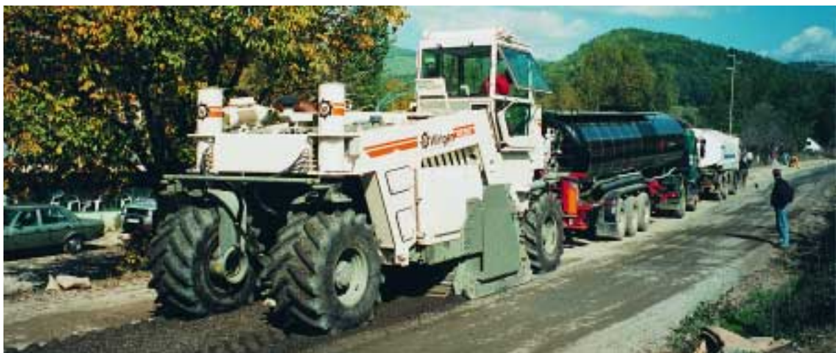
On this job site, cement was spread on the road surface prior to the WR 2500 starting its work. The machine's well dimensioned engine enables it to easily push the tanker trucks for hot bitumen and water during the recycling process.
