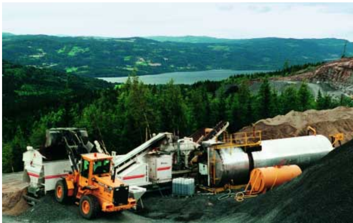
The mobile cold recycling mixing plant KMA 150 adds foamed bitumen to the pre-crushed and stockpiled aggregates and homogeneously mixes it with an hourly capacity of approx. 150 t.
