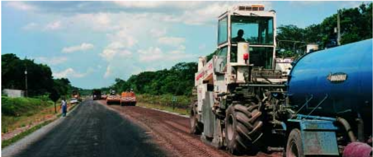
In South America, too, the Wirtgen foamed bitumen technology is gaining ground: In the air-conditioned operator's cabin, the machine operator is at ease even at extreme temperatures – as on this job site in Brazil.
