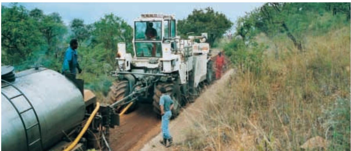
In this African Game Park, the network of traffic routes was rehabilitated with the WR 250 without disturbing the natural environment.
