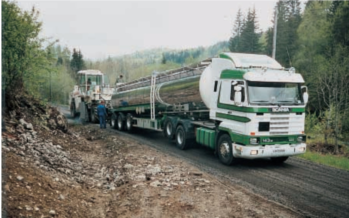
The WR 2500 demonstrating its power: On this job site in Norway, the store of binding agent in this bitumen tanker was sufficient for the rehabilitation of 2,500 m 2 in just under two hours.
