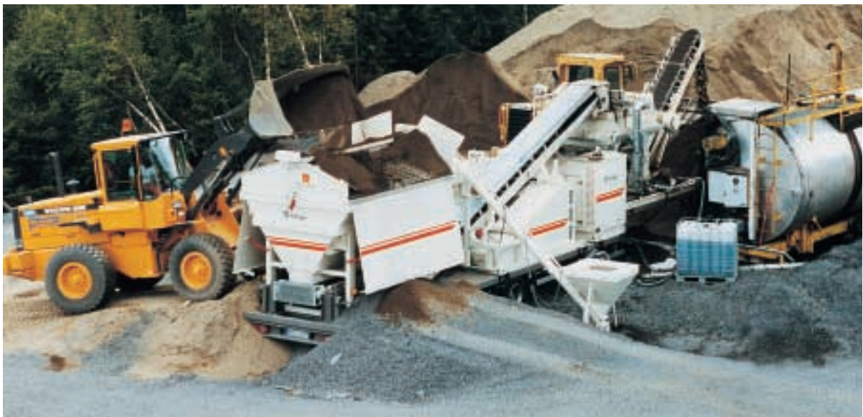
The Wirtgen Cold Recycling Mixing Plant KMA 150 can produce storable cold treated materials of the highest quality even in cold weather, with foamed bitumen being added as a binding agent: The mobile plant on a job site near Lillehammer in Norway.
