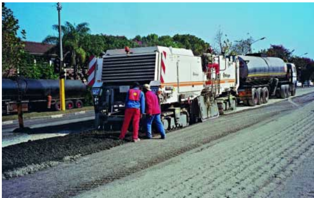
The road structure was recycled with the Wirtgen Cold Recycler 2200 CR to a depth of 20 cm and with foamed bitumen as a binding agent. The new base course was profiled by a grader.
