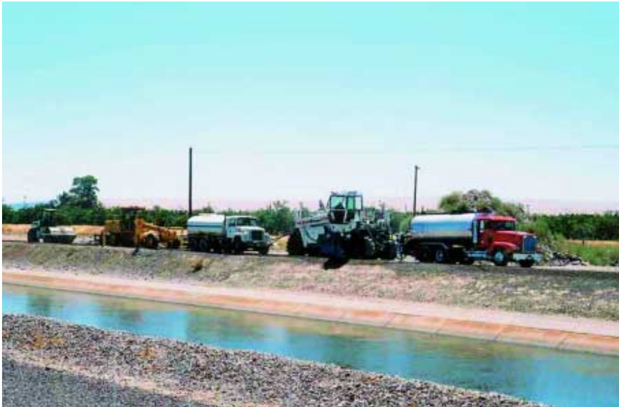
The recycling train including the WR 2500 working along the canal network in the Los Baños District. In future the canal roads can easily be trafficked again even with heavy-duty agricultural vehicles.
