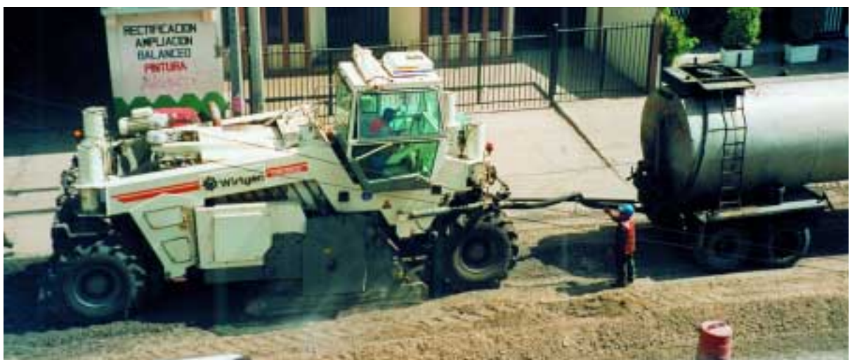
A rather cramped urban job site in Bogotá/Colombia: Here, too, the Wirtgen recycler WR 2500 feels at home and recycles the existing road structure swiftly and economically with foamed bitumen.
