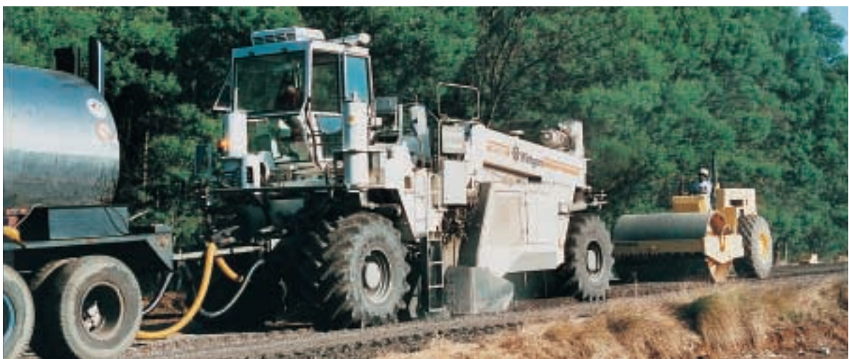
The rehabilitation of a traffic route in South Africa is an easy exercise for the WR 2500: Flexible hoses supply the recycler with hot bitumen and water which are sprayed into the mixing chamber in precisely metered quantities.
