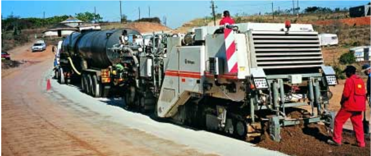
Reliable operation in South Africa during the rehabilitation of an urban road: The Wirtgen Cold Recycler 2200 CR is a machine that can be used for cold recycling as well as cold milling applications.
