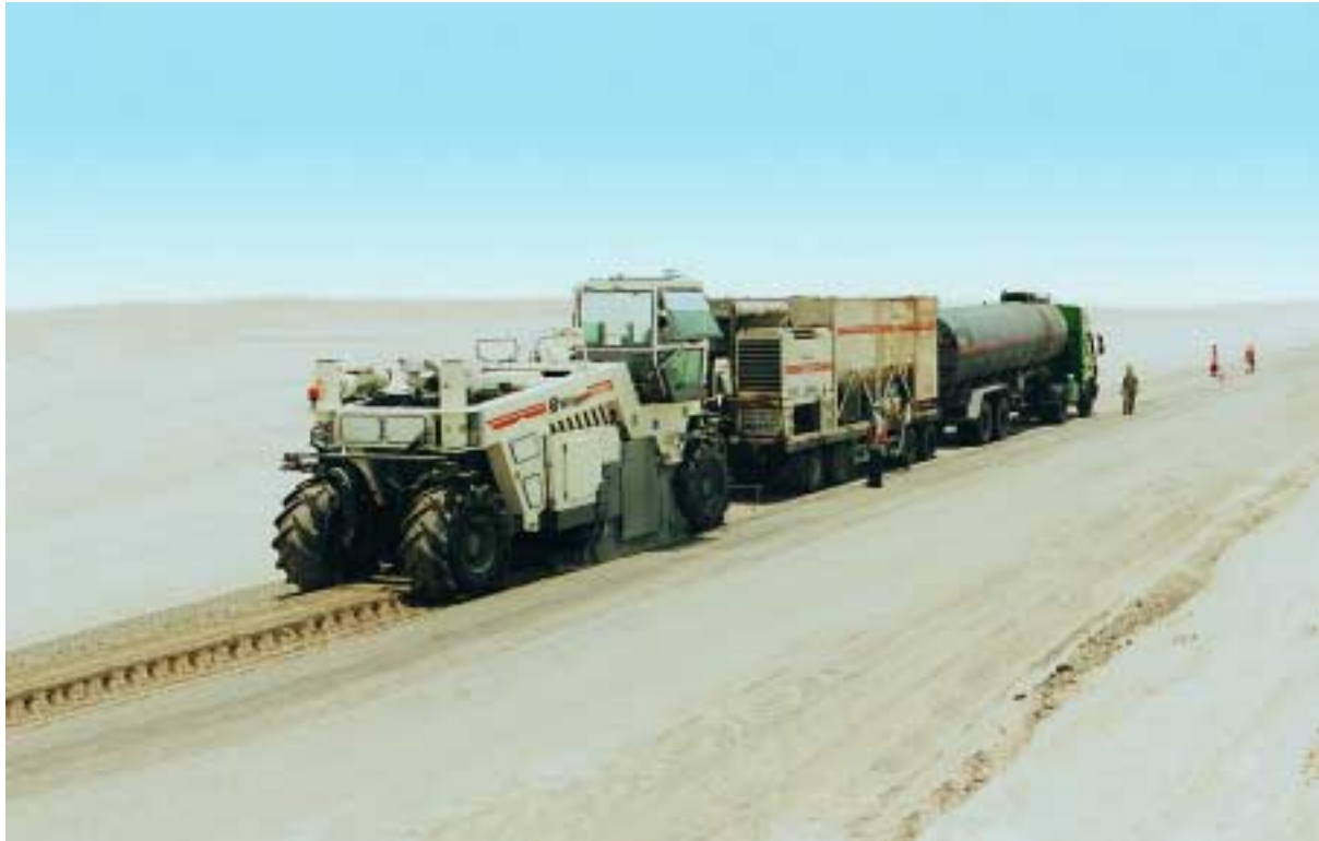
In operation 24 hours a day despite extreme climatic conditions: One of the three Wirtgen recycling trains consisting of a WR 2500 and a Slurry Mixer WM 400 during the economical rehabilitation of the Shaybah Access Road.
