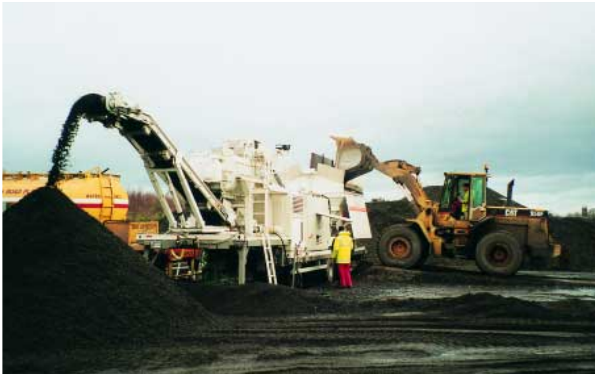
Stockpiling the milled material blended with foamed bitumen. Production of the KMA 150 can be started and stopped from the wheel loader via a remote control unit.
