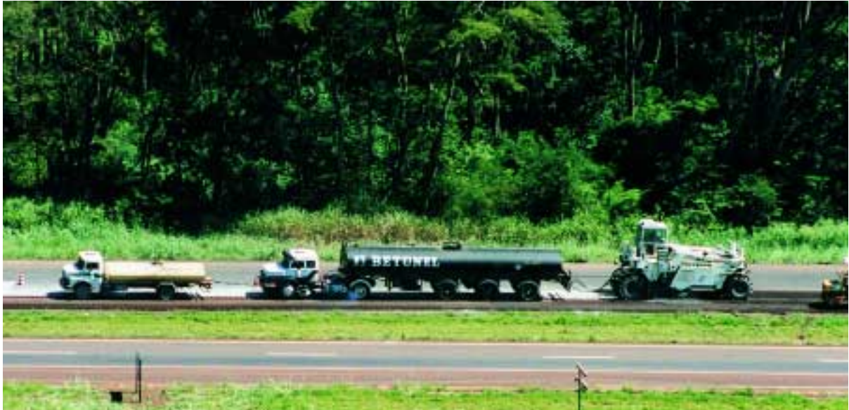
The Wirtgen Recycler WR 2500 impresses with optimum performance during a cold recycling application with foamed bitumen on a motorway job site in Brazil.
