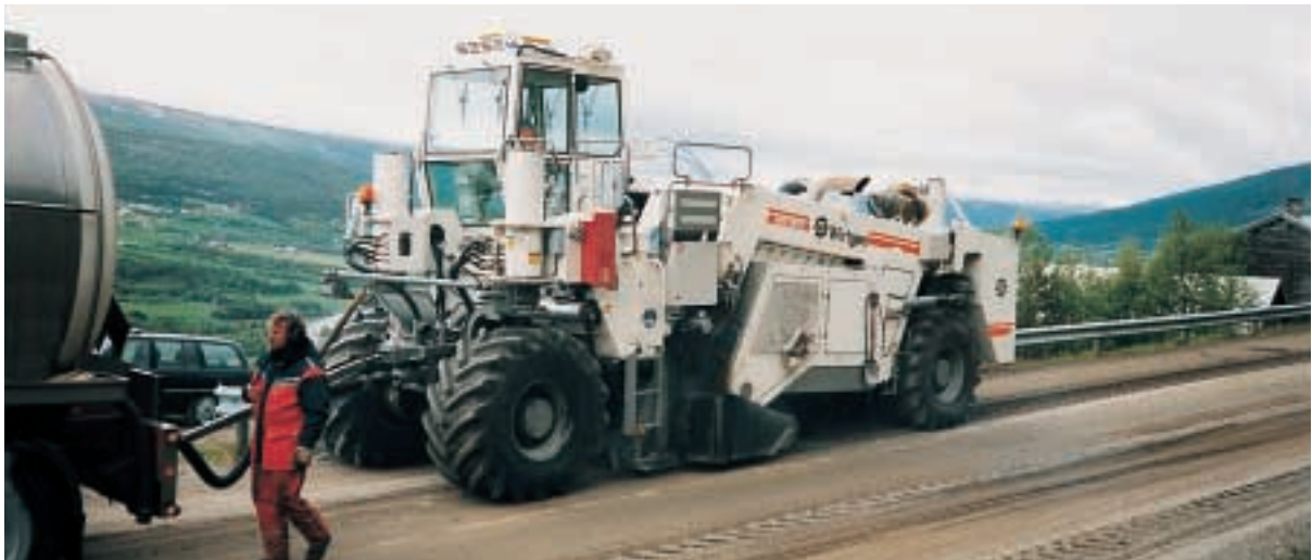
Road rehabilitation in Norway: The WR 250 is coupled to the insulated tanker truck, and hot bitumen is foamed and homogeneously mixed in the Recycler's mixing chamber.
